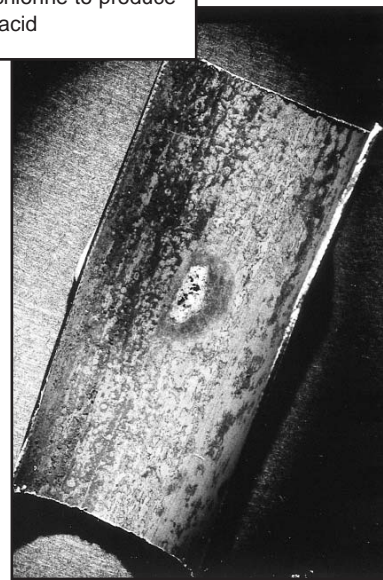
Figure 9: Crevice corrosion under bacteria colony on the inside of a stainless steel tube (magnification 5X)
